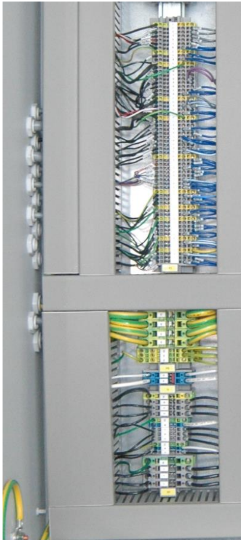
Figure 9: Terminal blocks with closed cable trays
